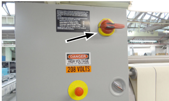
Figure 3-2: The main disconnect switch is located at the right rear of the unit.
