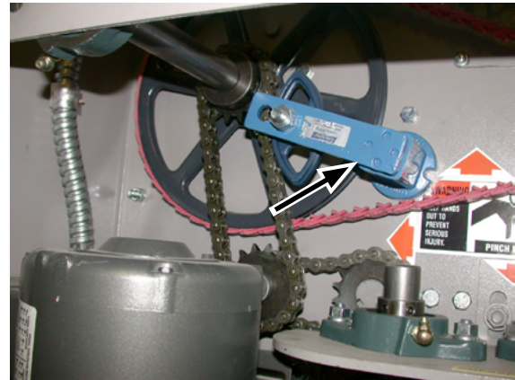
Figure 7-16: Tensioning idler arm in the upper left endframe.
